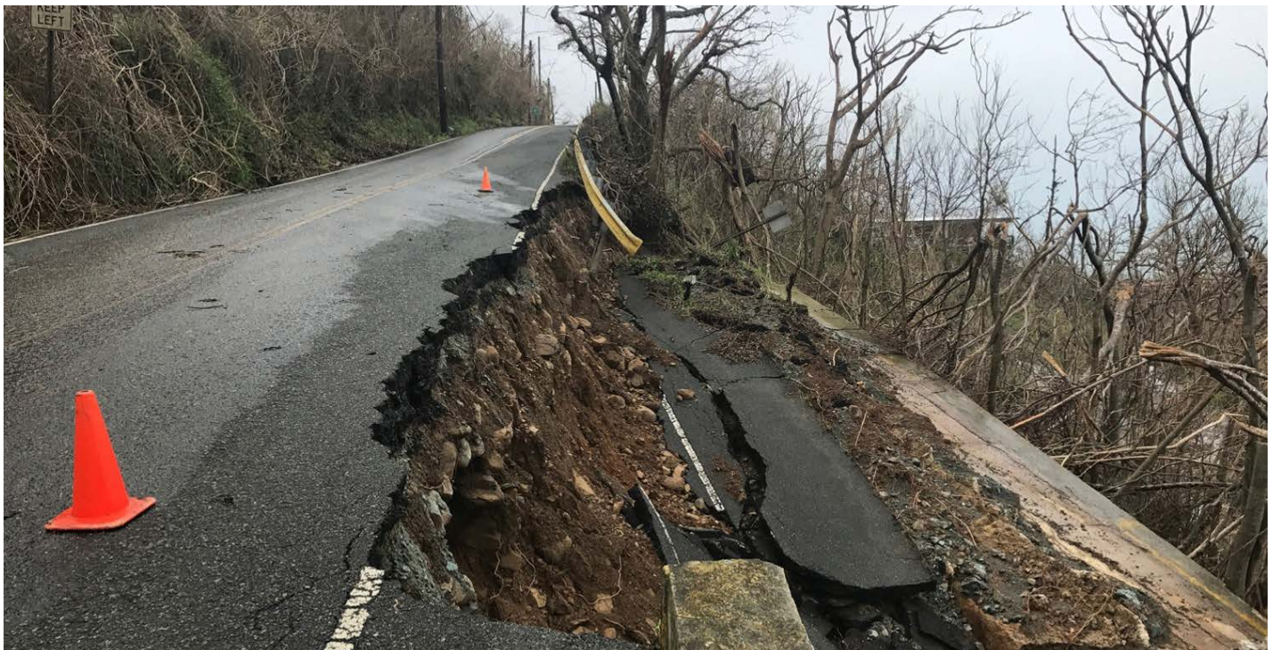
Hurricane damage to road in the USVI
