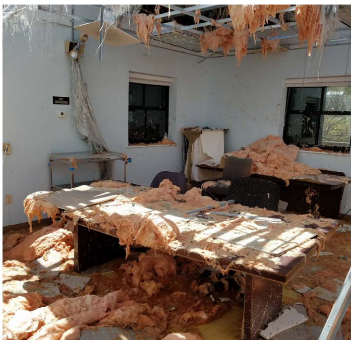
Damage to wastewater treatment plant, Mangrove Lagoon Geoffrey Watson/VIWMA
