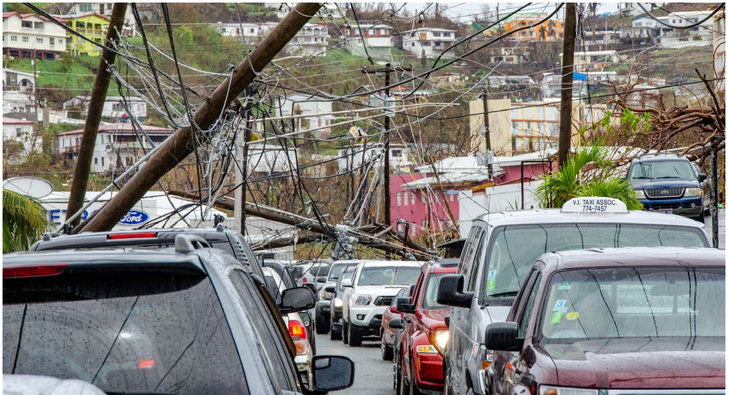
Hurricane damage to power lines on St. Thomas K.C. Wilsey/FEMA
