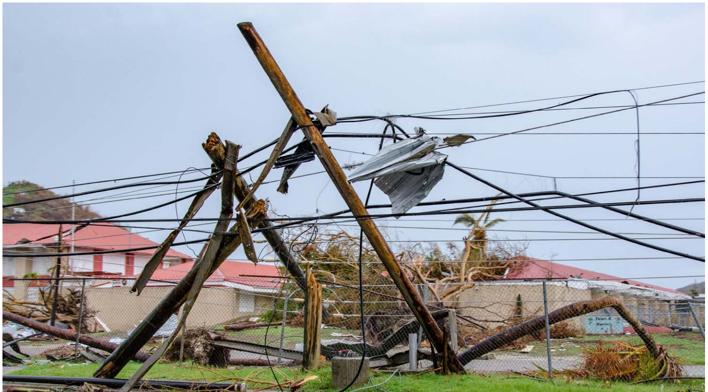
On St. Thomas, downed trees, snapped utility poles, and debris were evidence of the powerful winds from Hurricane Irma K.C. Wilsey/FEMA
