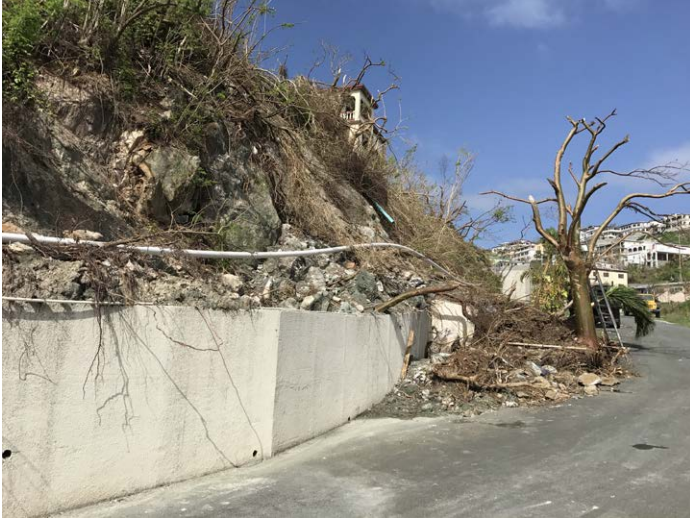
Damaged sewer lines at Anna's Retreat, St. Thomas VIWMA
