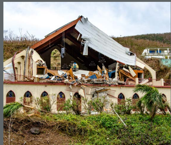
Hurricane damage to the Global Life Church on St. Thomas K.C. Wilsey/FEMA
