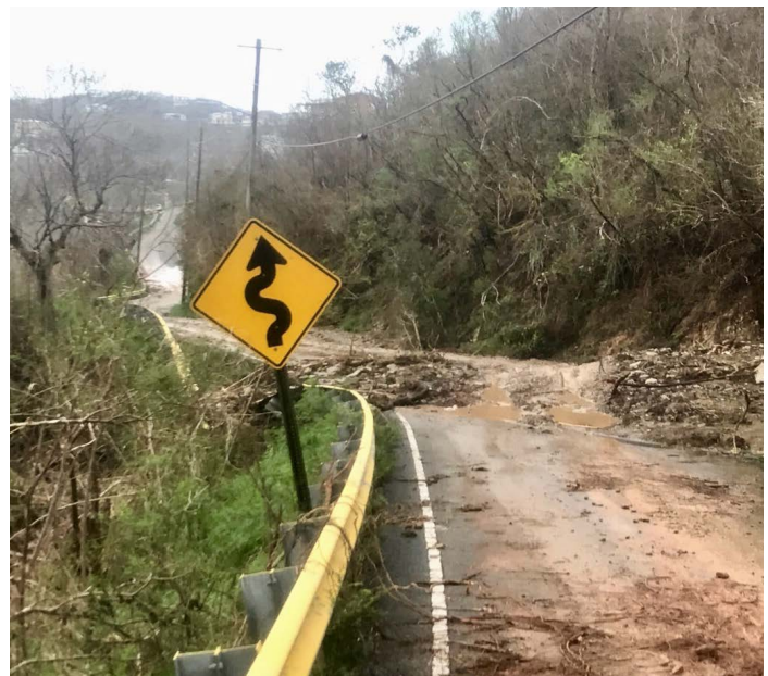
Damaged road on St. Thomas Kelsey Nowakowski
