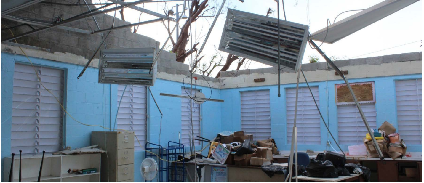
Hurricane damage to Gladys A. Abraham Elementary School on St. Thomas VIDOE
