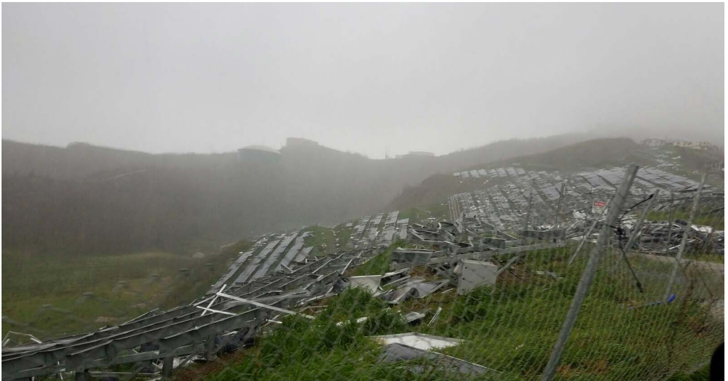
Damaged USVI 1 solar field on St. Thomas Kelsey Nowakowski
