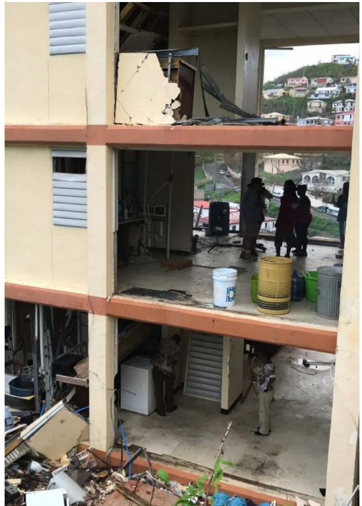
Residents in a damaged building cleaning up the remains Beth DeFalco
